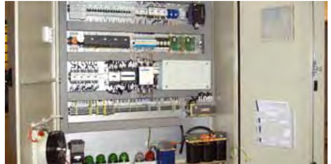
Maco B Magnet control cabinet
