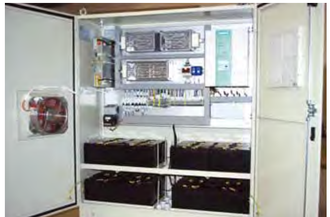
Emergency power system BBU
