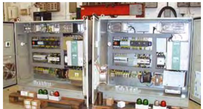
Maco EP Magnet control cabinet
